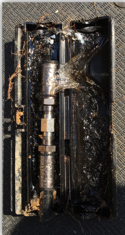
Figure 13: Opened Splice Enclosure with Water Ingress and Corrosion
