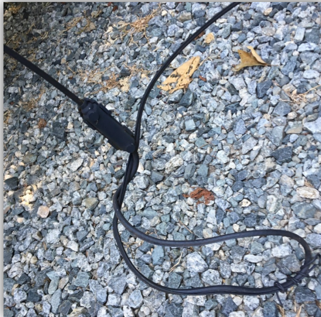
Figure 6: Inline Splice with Weather Enclosure
