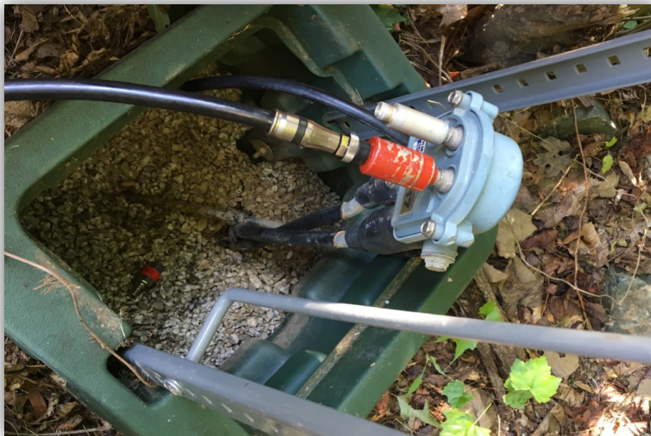
Figure 14: Bad Drop Trap Causing a Micro-Reflection
