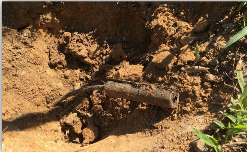
Figure 12: Buried Splice Enclosure with Series 11 Cable Pulled from F-Connector
