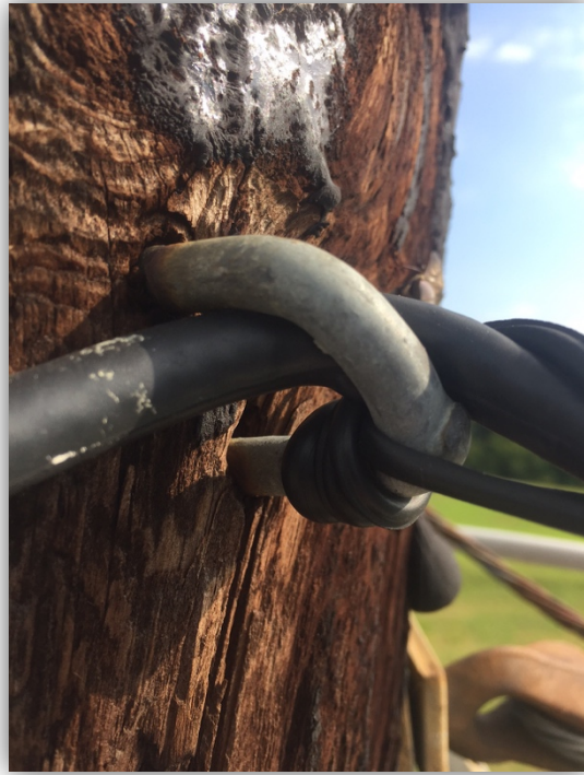
Figure 43: Drop cable looped around a j-hook connector causing the cable shielding to fail.
