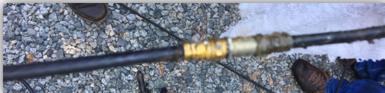
Figure 7: Corroded Crimp-on F-Connectors Exposed to Water
